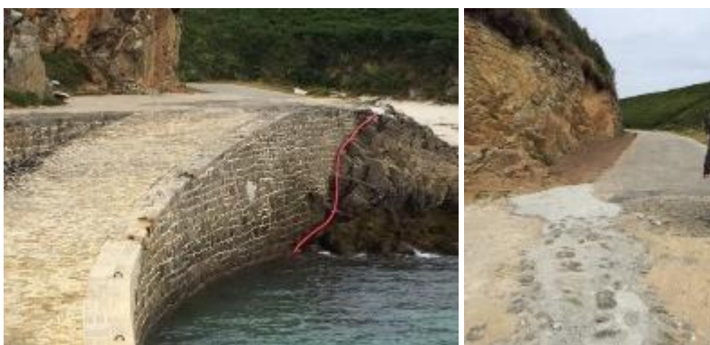
Figure 20: Passage of the cable past the slipway and along the cliff (SABELLA)
